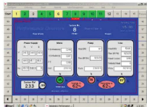
Dashboard for Pump Performance Monitoring
